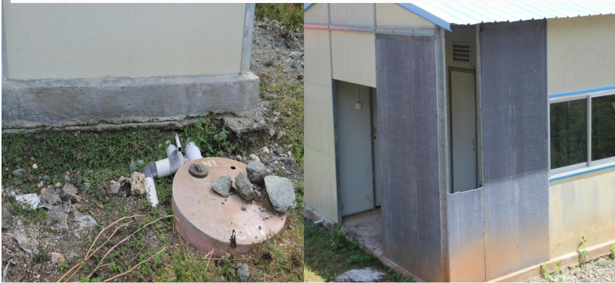
Photo 4; Some part of the community housing, such as septic tank and in certain wall of the building are destroyed.
