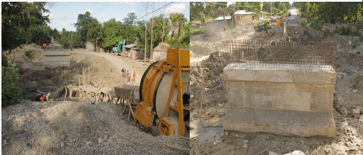
Photo 5; a bridge construction that categorized as emergency project in Asumaten sub-village has been interrupted for four months because of the contract has not exist yet. The company has stopped to continue the construction.
